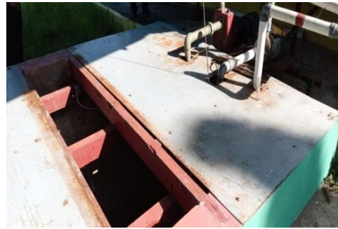
Gambar 2. Bak Inlet IPAL
