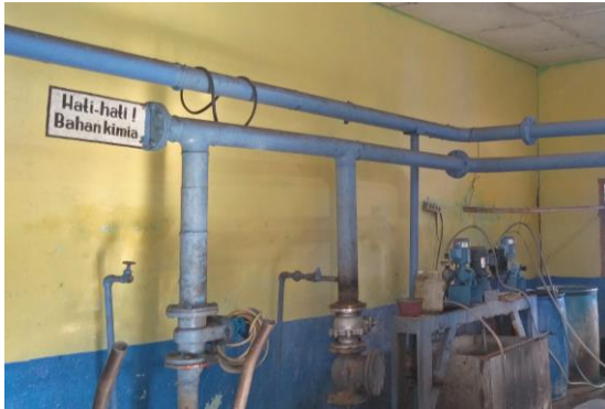
Stasiun Water Treatment Plant (WTP)
